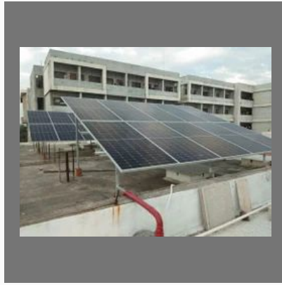
Solar Rooftop On Grid System
